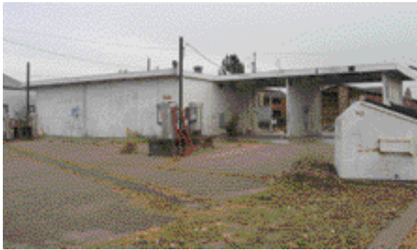
Before: Outdated and run down, the car wash was in desperate need of an extreme makeover.
